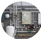
Panel Shops & Control Boards
