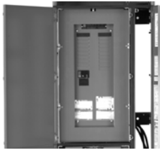
Distribution Panelboard in an MCC
