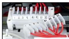
Control Terminal Block
