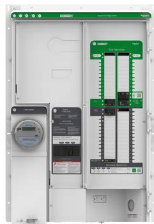
Energy Center with Cover Removed
